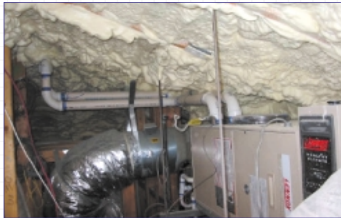
Icynene was sprayed on the underside of the roof deck to seal the building and convert the attic from unconditioned to conditioned space, thereby increasing the efficiency of the heating and cooling system.
